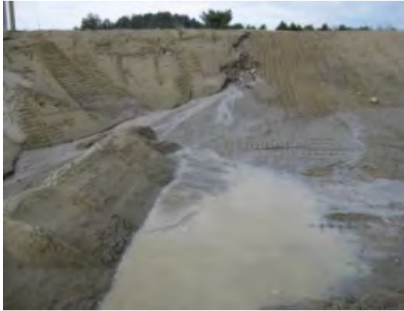
Seeping slopes are found at cuts that intercept the groundwater table. Often, riprap over a layer of drainage gravel is the only appropriate stabilization measure.
