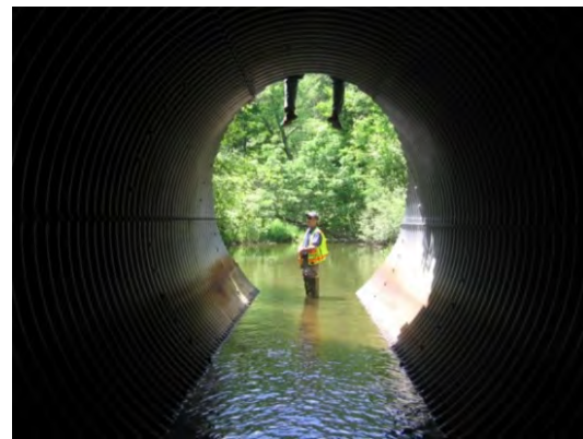
Inspect the structure after major rain events and repair immediately. Remove any debris that may block or constrict the culvert opening.
