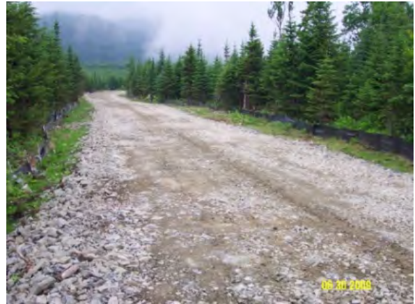
Good road surface and base material contains gravel, sand, and a few fines. Gravel and sand in the subbase provide strength and drainage.
