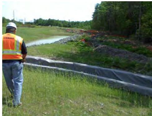
The slope drain structure should be inspected daily and during every storm event. The structure should be kept clear of sediment and debris.
