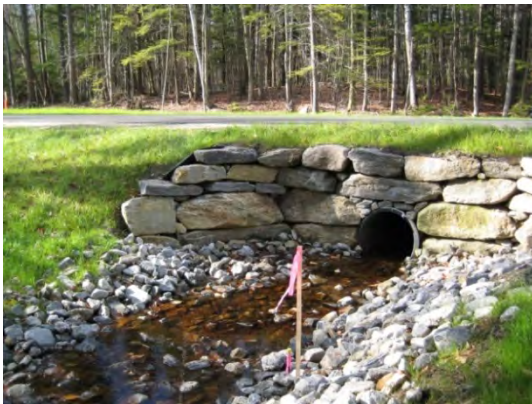
After installation, the streambed should be restored to its original shape and slope.
