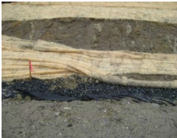
A continuous contact between the mat and the soil is critical, otherwise the mat may fail.
