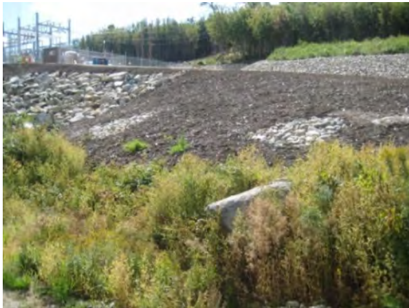
Groundwater drains, soil reinforcement or even a retaining wall may be necessary where the slope is failing due to groundwater seepage or soil instability.
