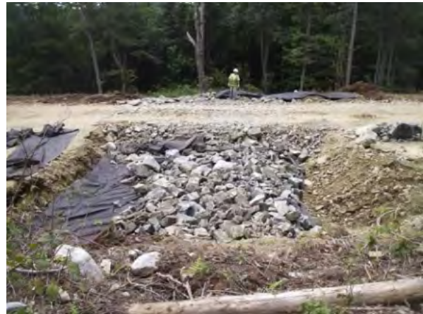
A rock sandwich can provide a permeable road base if built of coarse rocks and wrapped in geotextile fabric to let water drain downgradient.
