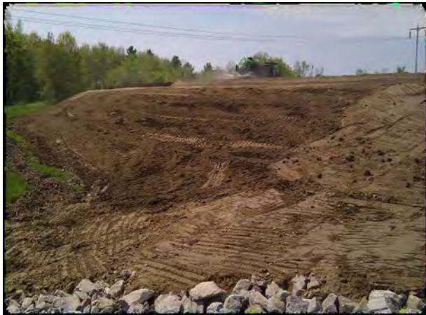
Soft sedimentary rock can be modified to create a surface for vegetation growth when the rock is rippable and can be shelved. The shelves will hold moisture, seed, and mulch.
