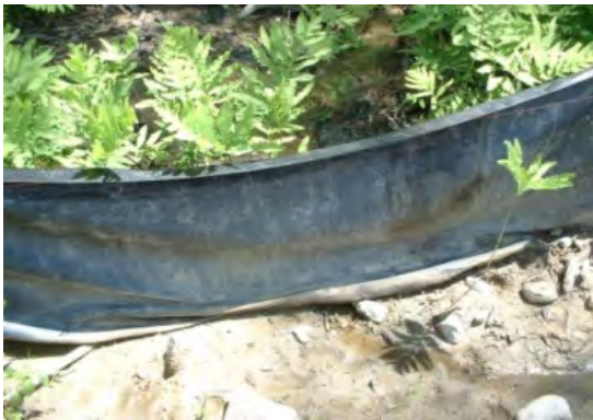
Silt fence can be difficult to install properly in shallow-to-ledge, stony, frozen, or forested soils.
