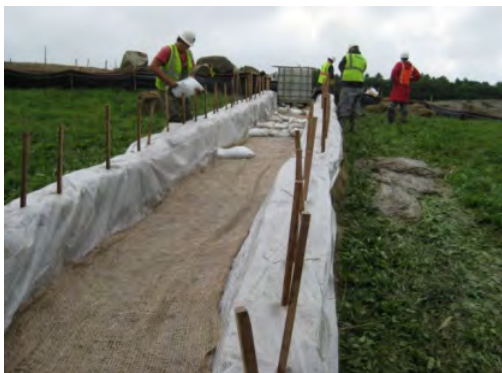
The slope drain should be located on undisturbed soil or well-compacted fill. Upon stabilization of the slope, a temporary slope drain can be removed.
